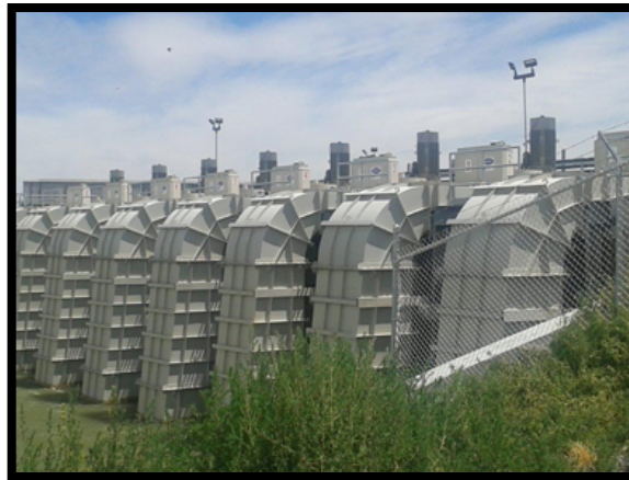
Eight Mavel TM10 Turbines Installed at North Side Canal Co.'s Head of the U Irrigation Project
